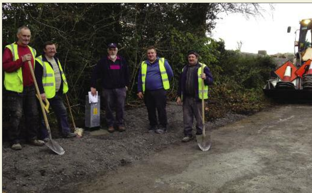
Boher Leamonaghan GWS in Offaly completed installation of bulk meters at strategic locations on the network.
