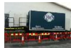
QWS Mobile Pumping Unit
