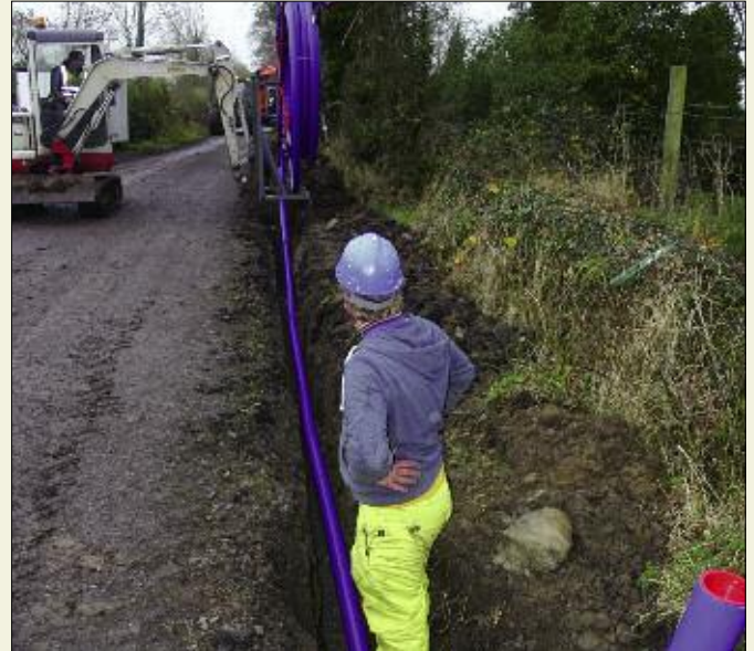
Full marks to the contractor replacing critical mains on Mid Roscommon GWS who fabricated a frame for 100 metre pipe rolls. This allows pipes to be laid smoothly and evenly in the trench without being dragged.
