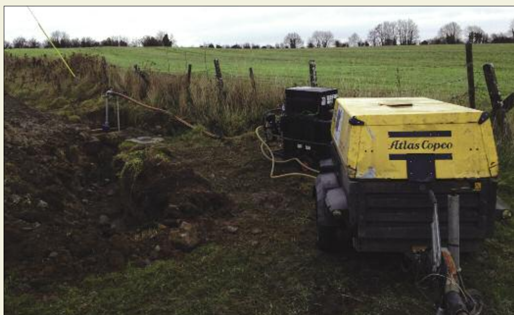
Air scouring was employed as part of a comprehensive network cleaning programme conducted by Lacka GWS in a successful initiative to remove manganese deposits from the internal lining of pipes.
