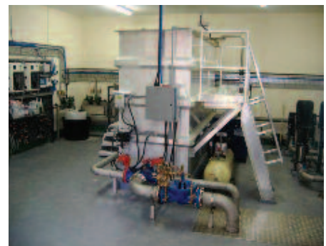
Castlebaldwin WTP, Co. Sligo
