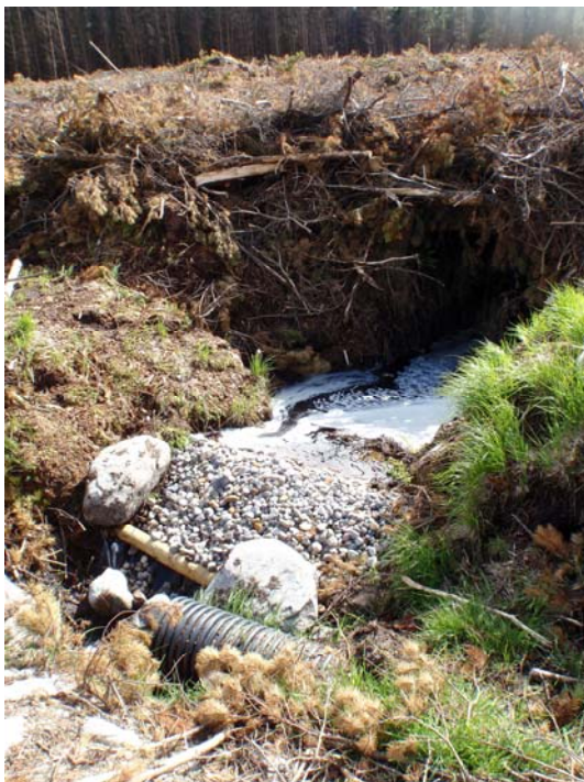
Figure 6.8 Permanent silt trap, preceded upslope by a settling pond.
