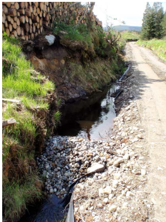
Figure 6.9 Permanent silt trap on road side drain.
